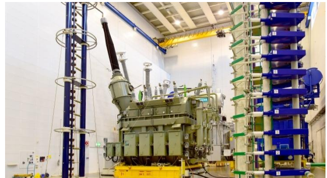
Synthetic-ester-filled power transformer in the test bay.
